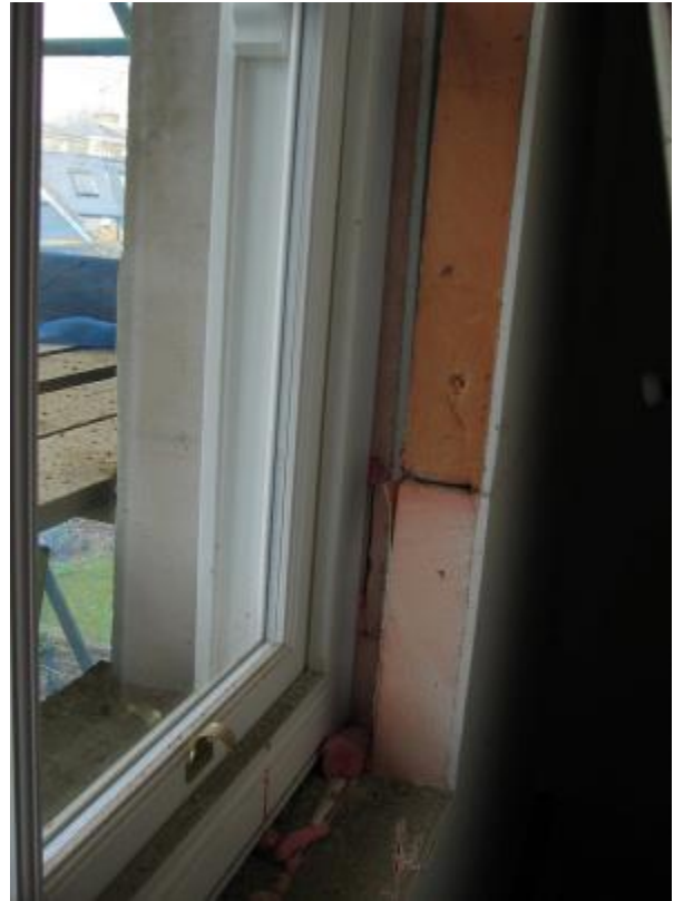
Figure 2 New timber double glazed sash windows and internal wall insulation in a Victorian house
