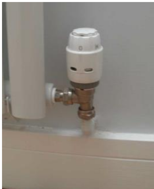
Figure 3 - Thermostatic Radiator Valve (TRV)
