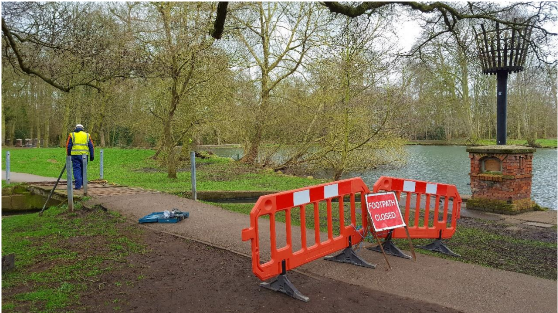
The Beacon at the Lake during renovation works. Photo: Boutham Park Digital Archive.
